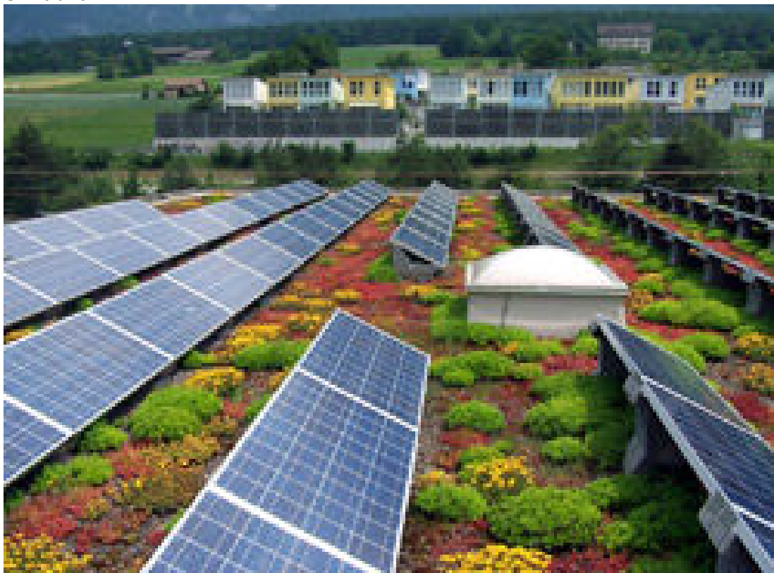
Sedum roof with Photo voltaic panels
