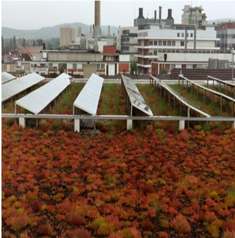
Brown roof with photo voltaic panels
